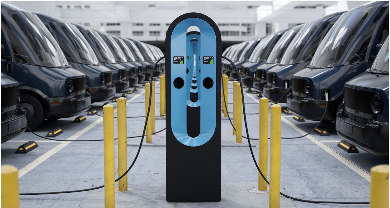
Electric EV delivery vans are being charged in a company parking garage
