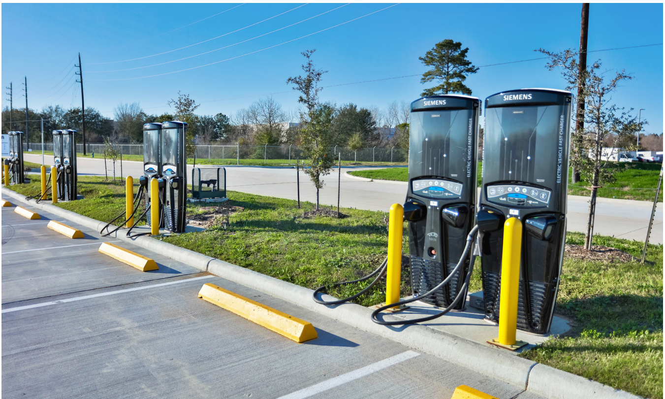
Charging stations at a Houston distribution facility
