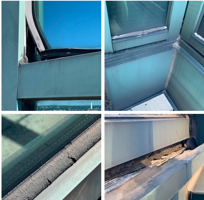
Curtainwall façade deteriorated conditions
